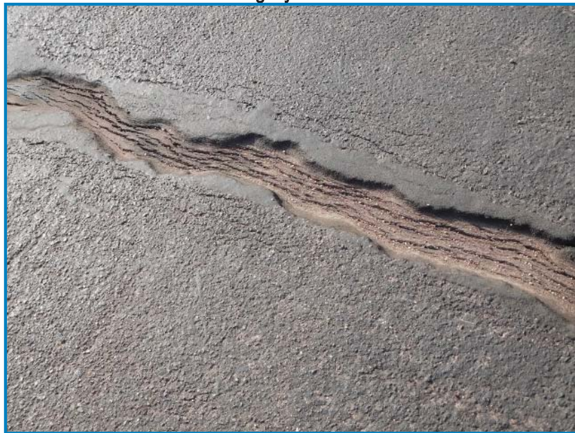
Asphalt cracking noted
