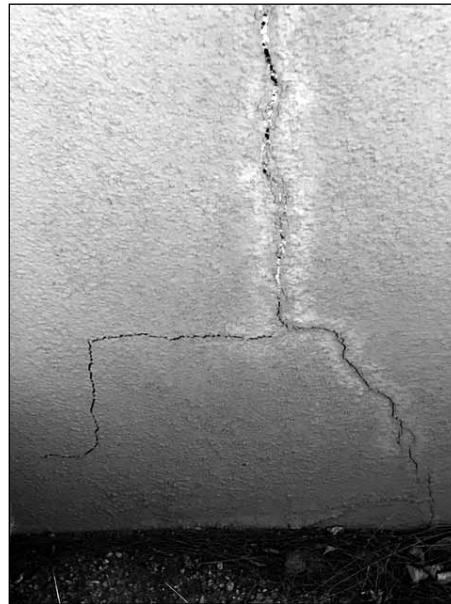
This stucco wall in High Desert has been damaged from excessive waterflow leaking into the inner wall.
